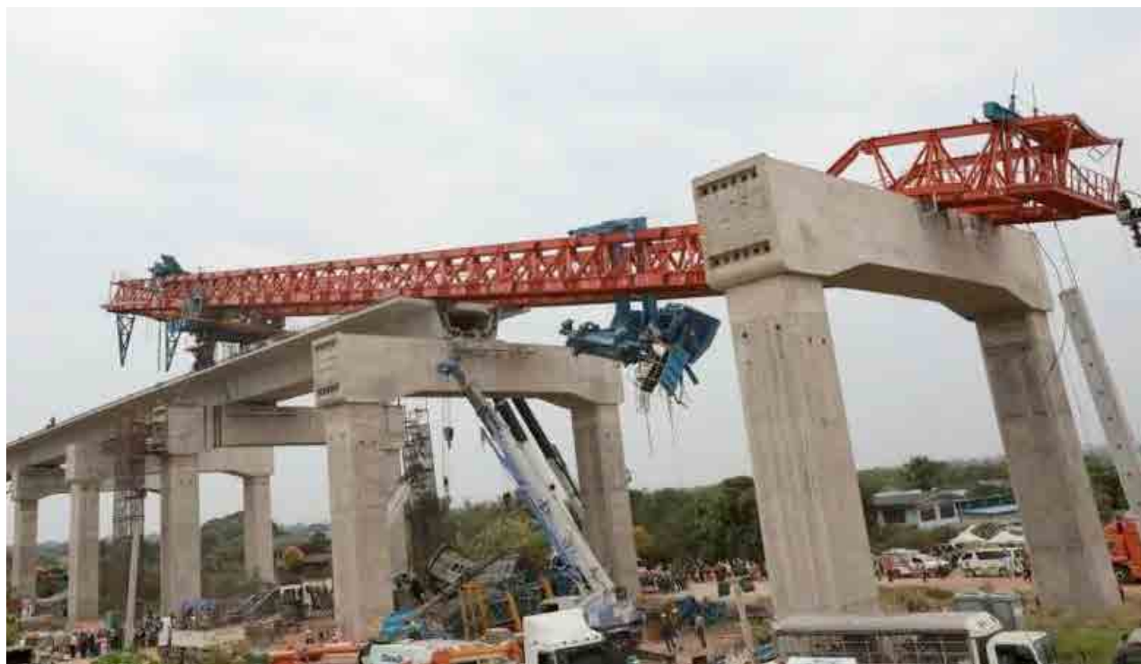
CRANE COLLAPSES ON TRAIN:
