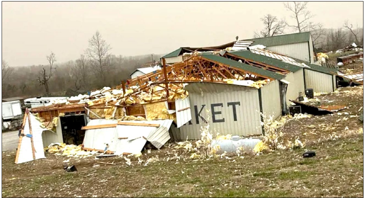
TORNADO: Damage from a tornado that hit Missouri.
