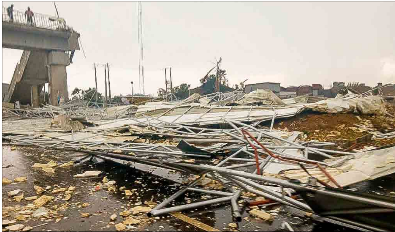
RIPPED OFF ROOF:
