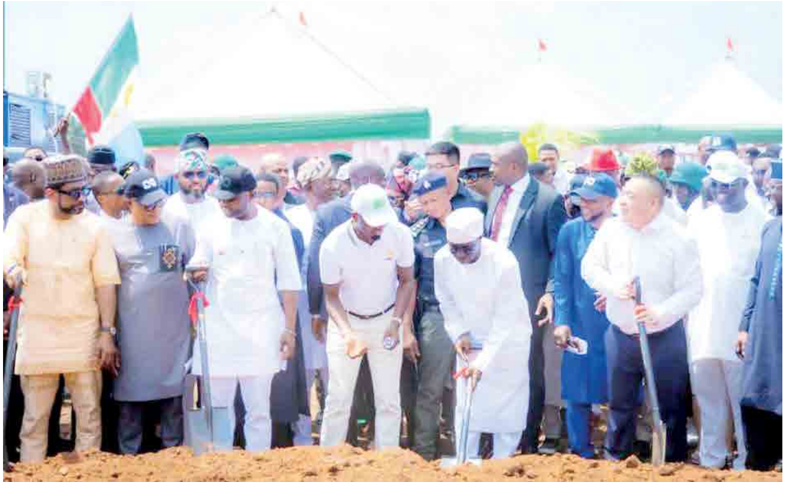
Edo State Governor, Senator Monday Okpebholo Launches 100MW Power Plant and LNG Facility at Ologbo in Ikpoba-Okha Local Government Area of the State performing a groundbreaking ceremony for the establishment of a 100MW Power Generating Plant and 300 Metric Tons Per Day LNG Facility, Taihu Industrial Park in Ologbo.
