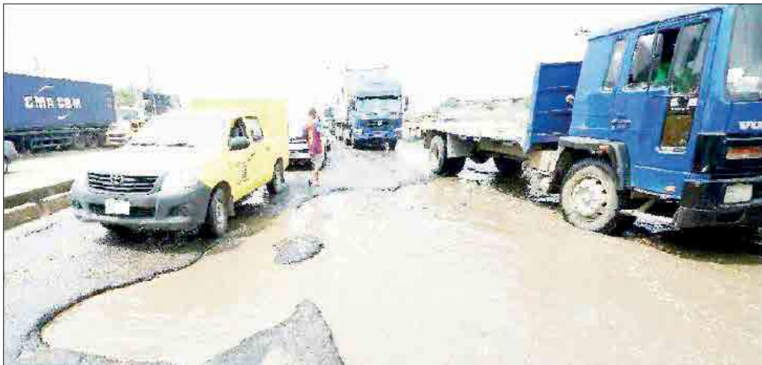
FEDERAL ROAD POTHOLE
