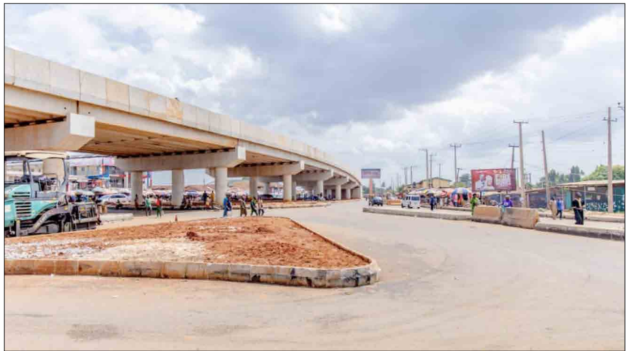
SIGNATURE INFRASTRUCTURE: The nearly completed Ramat Park flyover bridge constructed by the Governor Monday Okpebholo administration to transform transport and commercial activities in Benin metropolis.
