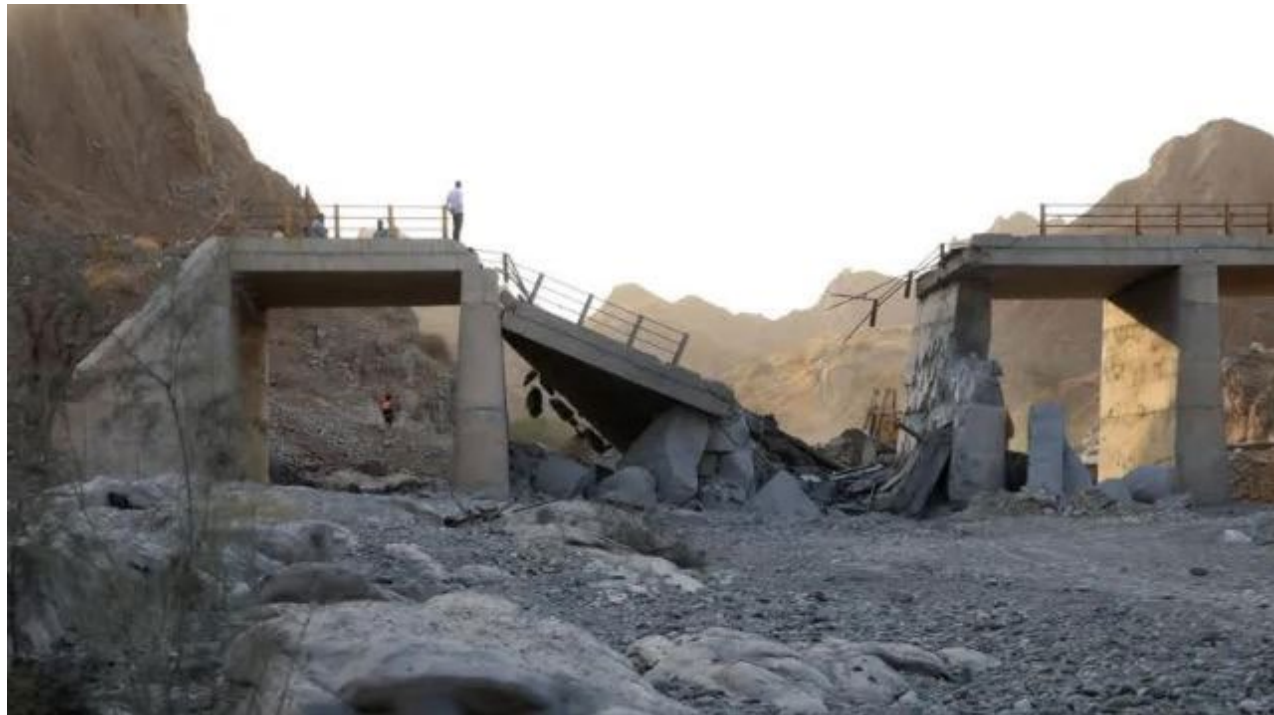
IRAN BRIDGE DAMAGED:
