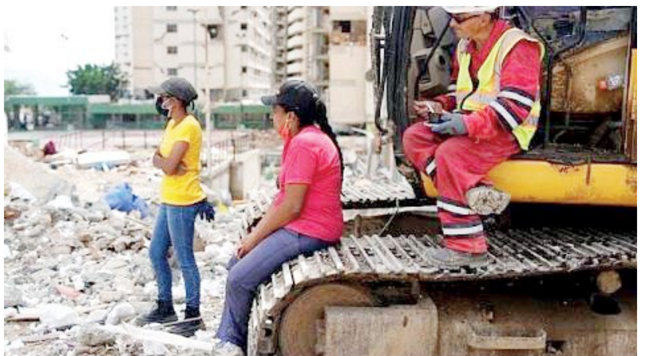
VENEZUELA COLLAPSED BUILDING:
