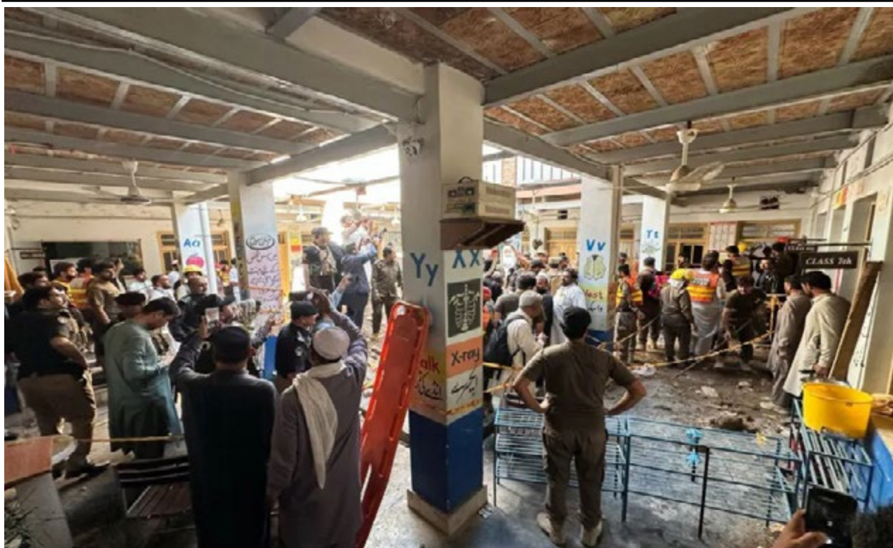
RESCUE WORKERS AT THE FIRST-FLOOR ROOF WHICH COLLAPSED INTO A GROUND-FLOOR CLASSROOM BELOW, CAUSING ITS CEILING TO CAVE:
